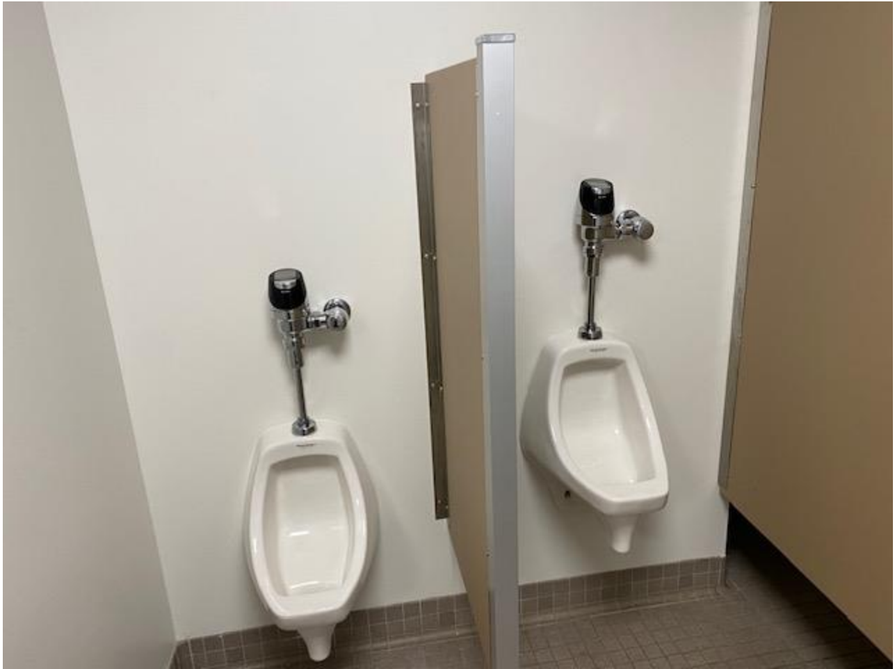
This is an existing bathroom in the firehouse. Notice the lack of tile on the wall behind the urinals.
