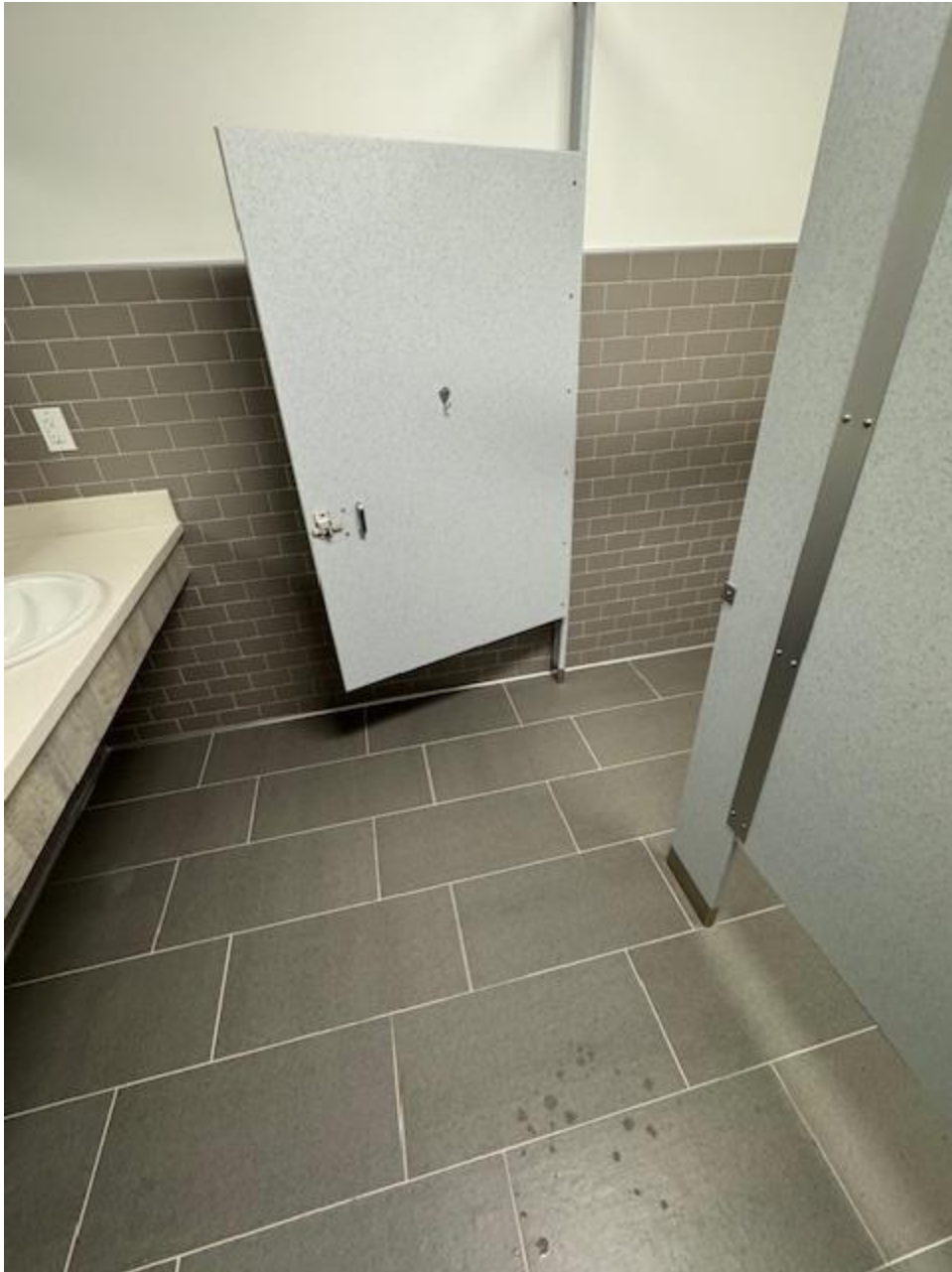
This is an example of a bathroom located in the Rec Center. Notice the tile on the walls.
